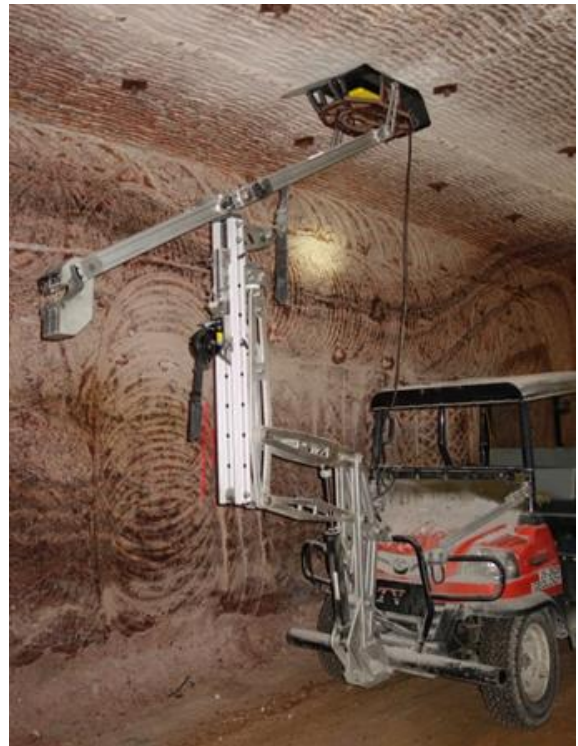
Fig. 2. The GPR-RTV used in the Picadilly mine. A 500 MHz antenna is mounted on the lift.
